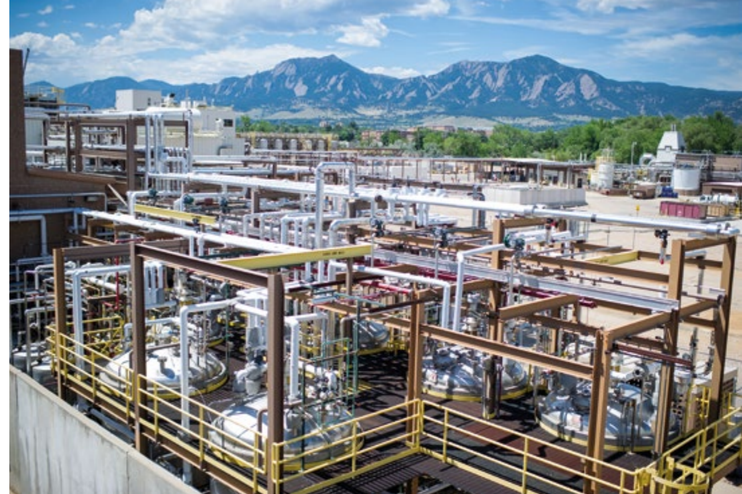
CordenPharma Colorado (USA) solvent handling infrastructure to support small molecule manufacturing.
